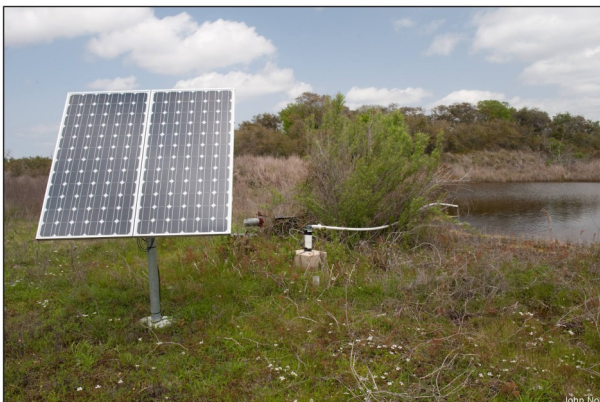
Moreno - Blackjack Peninsula - Solar Panel and Pump - 3/27/2010 1:27:36 PM
